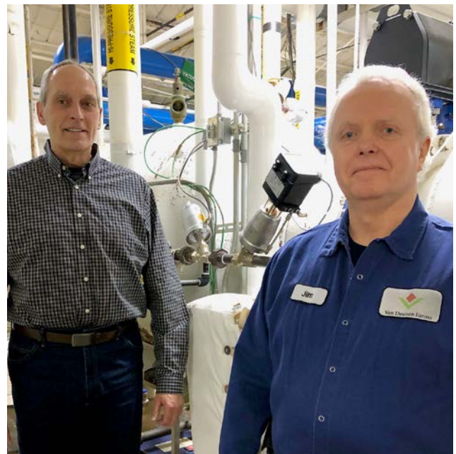
Rick Ouwenga (l) and Jim Leeneman (r) with 7010 and 7020: "These valves provide us with multiple economic advantages – both in terms of the process and the operating and maintenance costs."
