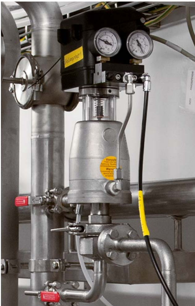
Fig. 2 The right-angle valve of the series 6000 from Schubert & Salzer Control Systems in the Okotberfest-container facility of Paulaner.
